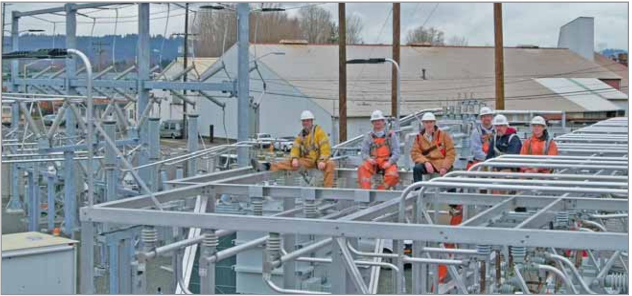
Cowlitz PUD's substation crew sits atop the newly rebuilt Seventh Avenue Substation in Longview, prior to it being re-energized in early April when construction was completed. The substation was rebuilt to help serve load growth in the area, which included a conversion to 115 kilovolts. JH Kelly of Longview did the civil construction work to clear and prepare the site and the PUD substation crew built the electrical structure. PUD relay and line crews and wiremen also worked on the project. This is the fifth PUD substation built or rebuilt in the last four years as part of our long-term infrastructure improvement plan. Next up is the John Street Substation in Lexington.
